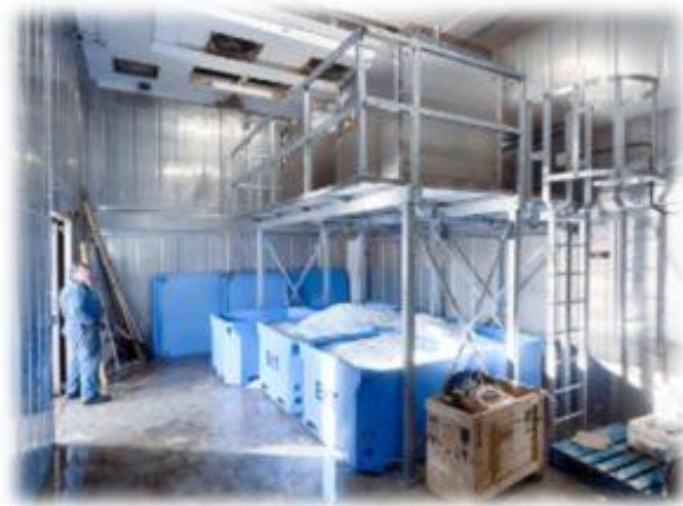
Inside the new ice facility, 2020
